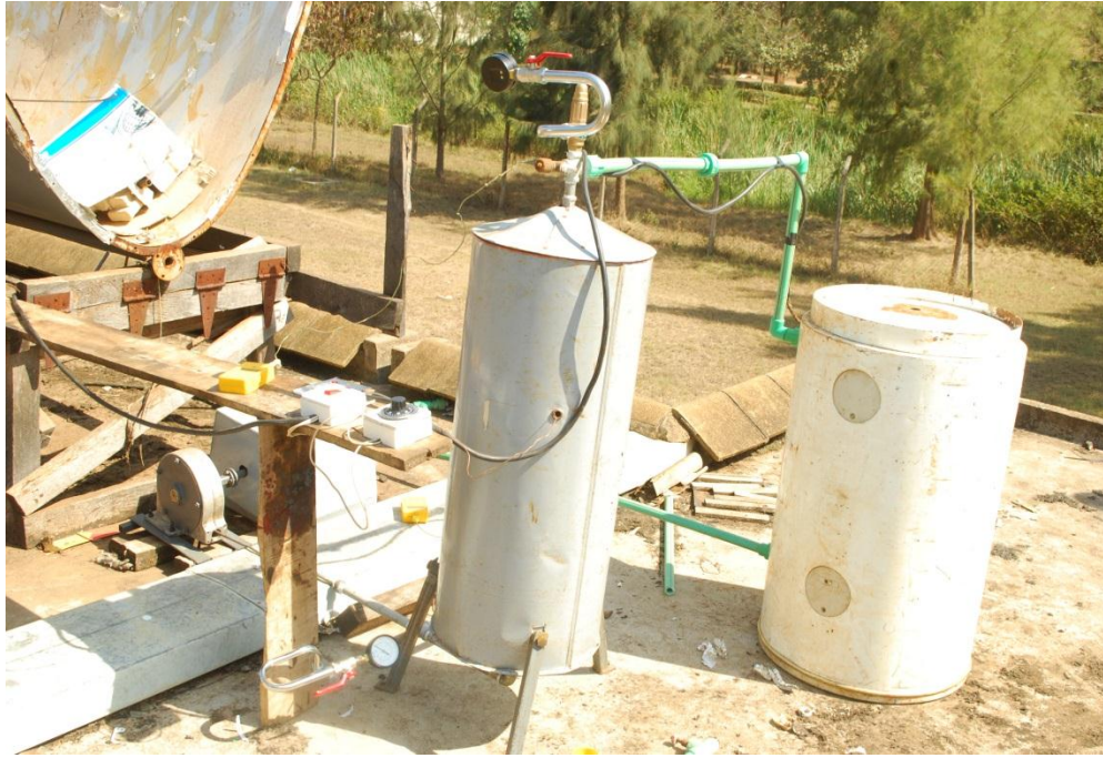
Plate 2: Steam storage system testing
