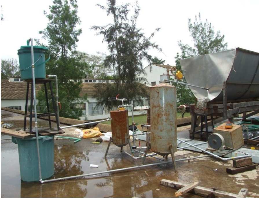
Plate 13: Solar thermal collection for salt solutions and unused engine oil
